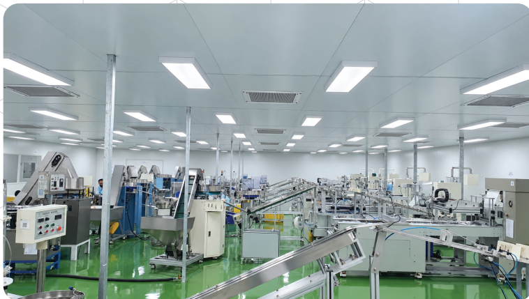
Production Room - ISO 7 Cleanroom
