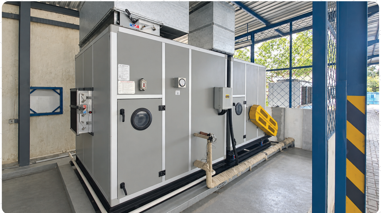
Air Handling Unit 65 RT
