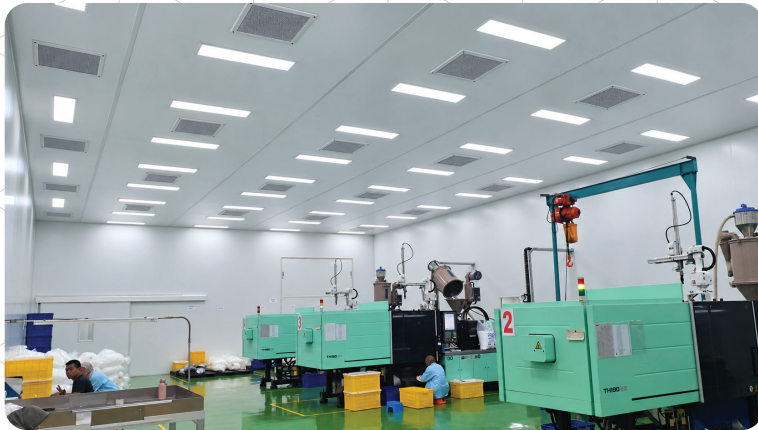
Injection Room - ISO 8 Cleanroom
